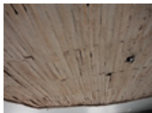
Area of fallen plaster.
