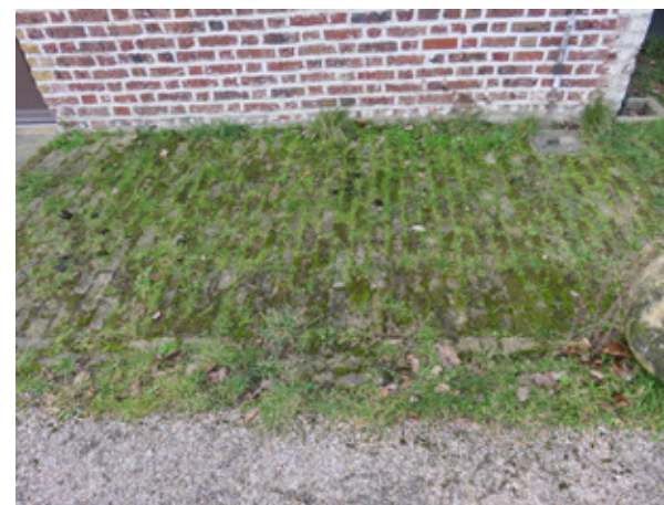
Figure 91 Vegetation growth on the brick paving at the rear
