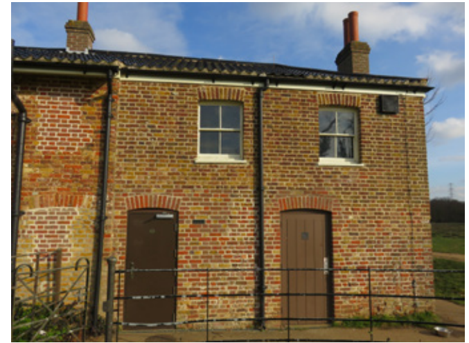
Figure 90 The estate railings have failed paintwork partly because they are climbed on, especially near the WCs
