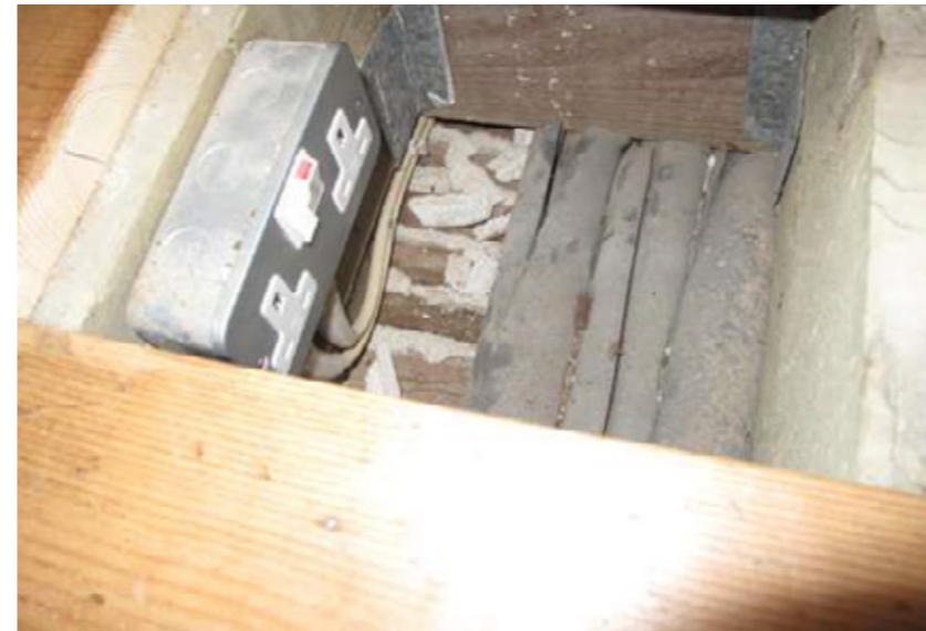
10. View into access point showing plaster debris from damaged key to timber
