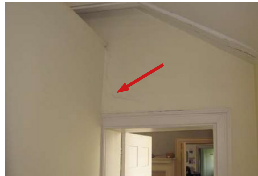
8. Upper ground floor; crack to finishes
