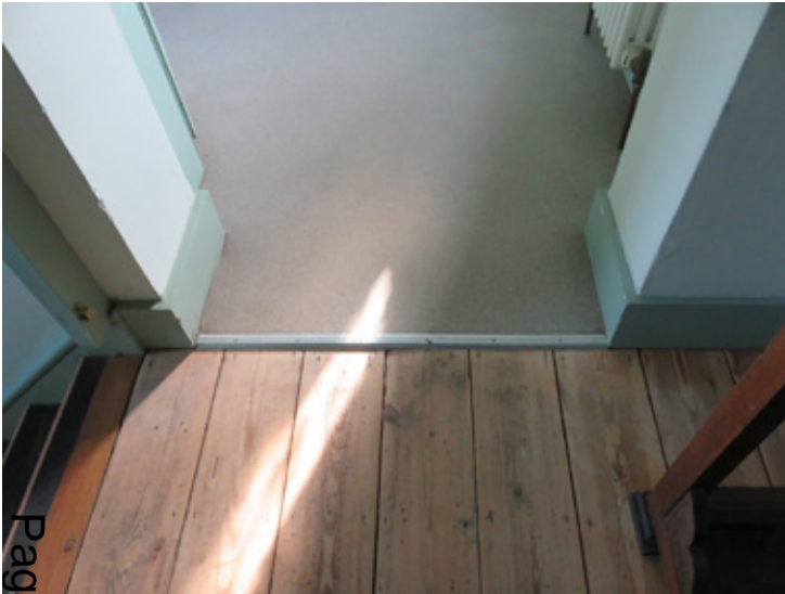
Figure 15 The threshold between the small early 19th-century extension and the later 19th century recessed extension on the upper ground floor.
