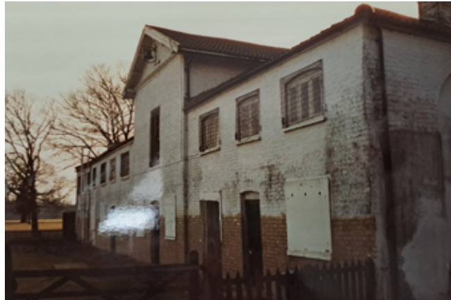
Figure 66 A photograph taken of the east elevation during the removal of the white render. City of London Corporation, HB/TEM/16
