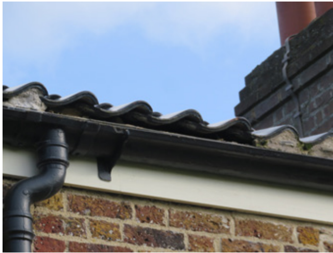
Figure 86 Failed mortar ends to the roof tiles
