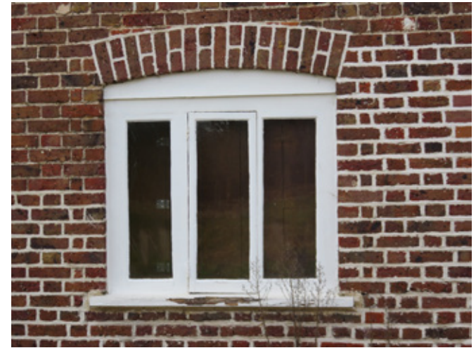
Figure 87 Rotting window cill
