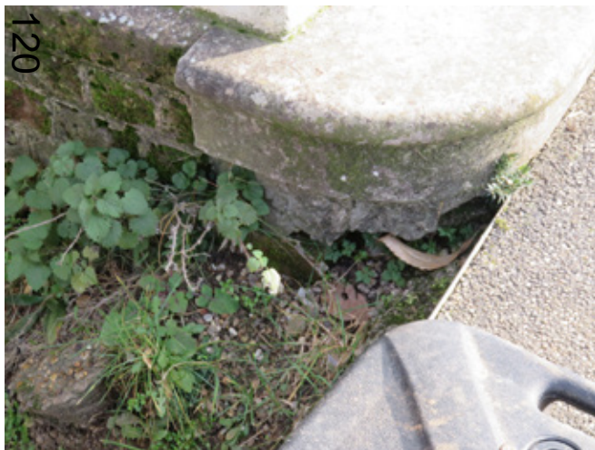
Figure 88 Erosion under the main steps
