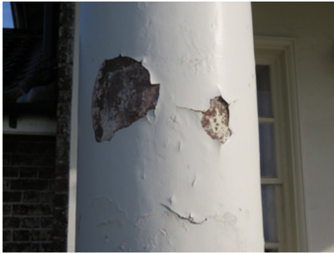
Figure 89 Failing paintwork to the columns
