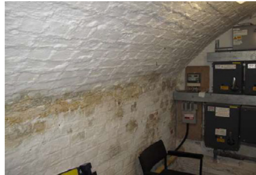
7. Vault below entrance portico showing areas of water ingress
