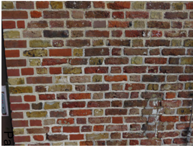
Figure 85 Some of the pointing is drude and there are small areas of cementitious mortar
